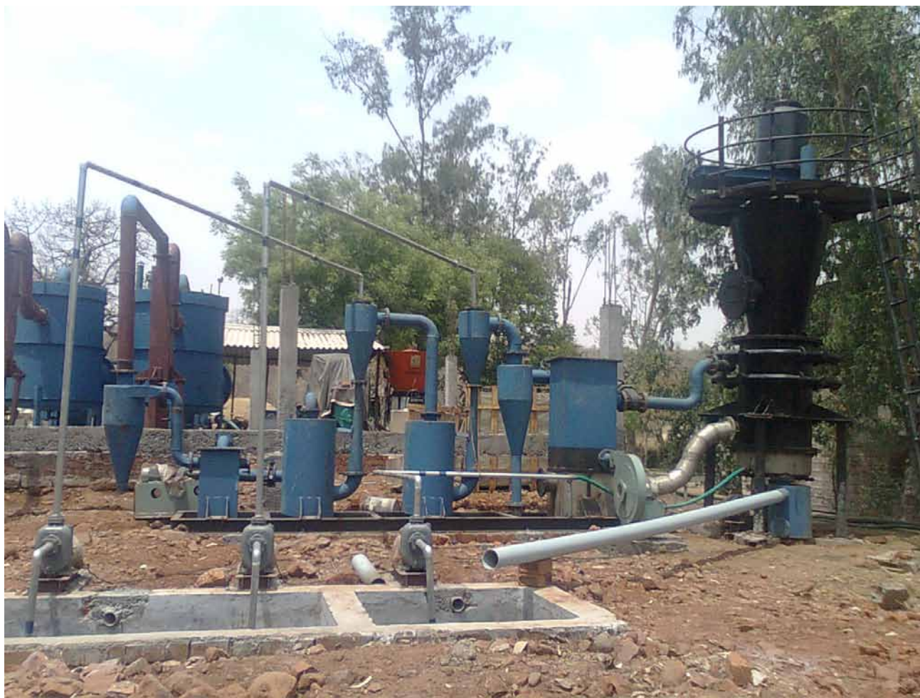
Panoramic view of gasifier system
