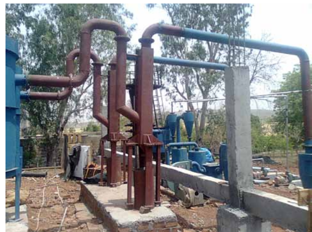
View of gas dehumidification unit
