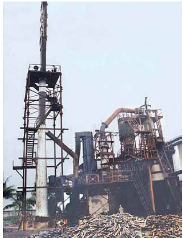
Venturi scrubber system, Howrah
