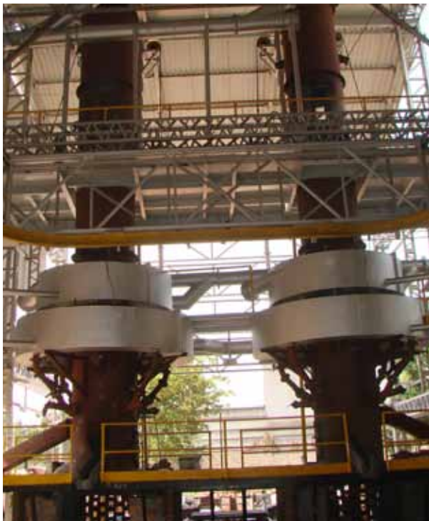
DBC commissioned at Aquasub Engineering, Coimbatore
